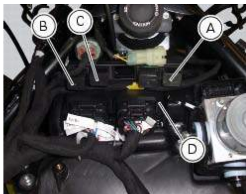
A injection relay; B ETV relay (throttle valve actuator motor), C radiator fan relay, D engine control unit.
