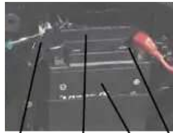
positive wire strap battery negative wire
