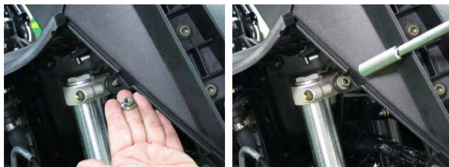
Install the two nuts mounting on the front cover meter on both side.
